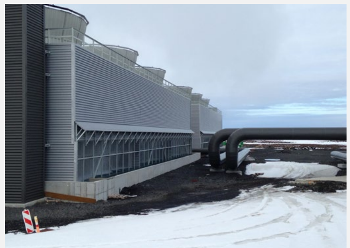
Cooling tower in Iceland
