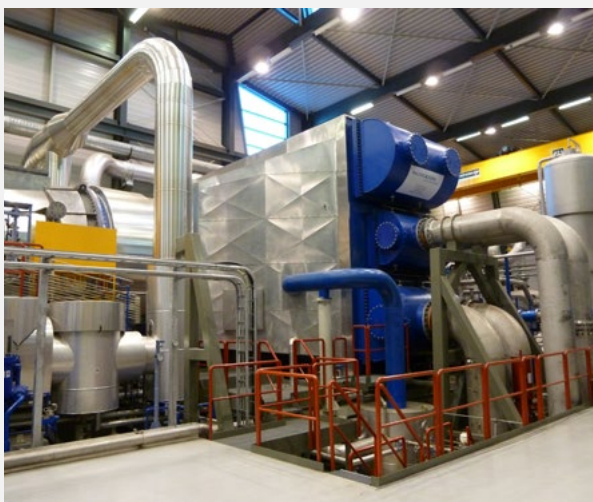
Surface condenser inside a power plant in Iceland
